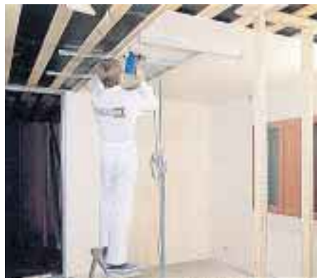
When using mechanised screw insertion the penetration of the screw head into the board can be set to the desired depth (with boards to be filled it should be approx. 1-2 mm).
