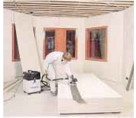
During the cutting operation, the guide rail rests on the panel by adhesion. A suction unit operates at the same pace with the saw extracting chips and dust into a bag.
