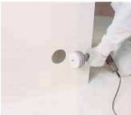
A cut made with a power drill is neat. The tight fit meets the requirements of sound engineering and the sockets are installed securely on the wall.
